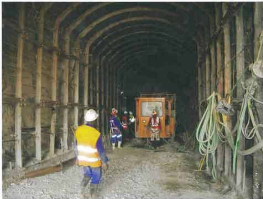
The Yalou mine in Mali, where Shaft Sinkers is sinking a 4,5 m x 4,5 m twin decline system (photo: Randgold Resources).
