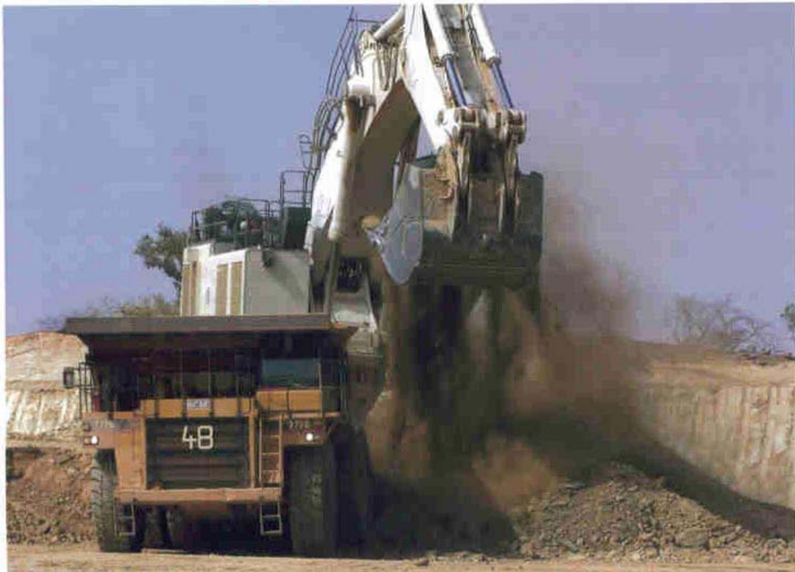
Site preparation at Randgold Resources' Yalea underground mine at the Loulo complex in Mali.
